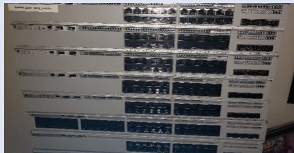
IMAGE OF NEW CISCO 9200L LGBPS SWITCHES
